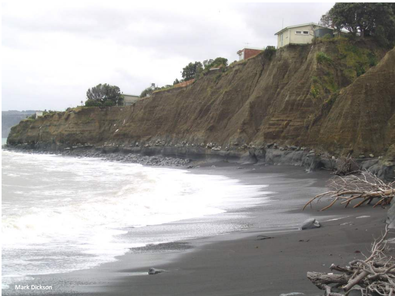
Figure 2. Housing threatened by coastal erosion, Cape Palliser Road, Wellington.
