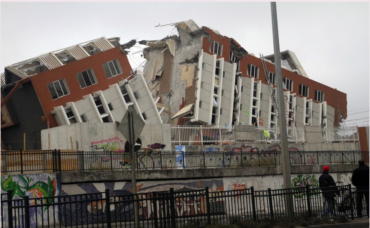
A building in Concepción destroyed in the 2010 Chile earthquake. Credit: Claudio Núñez CC BY-SA 2.0
